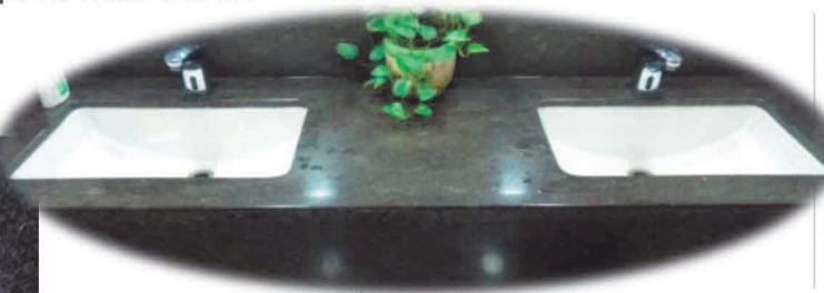
Water sensor taps in wash basins
