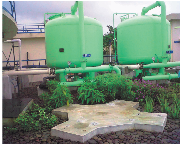
Pressure Sand Filters
